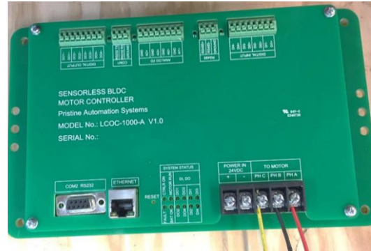
Conductor Cable Termination on Controller
