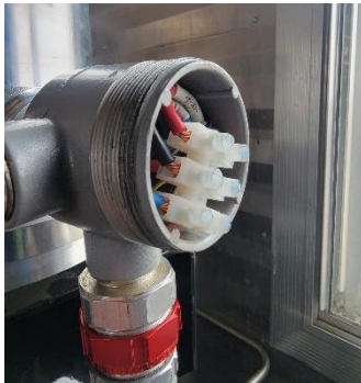
Conductor Cable Termination in Junction Box
