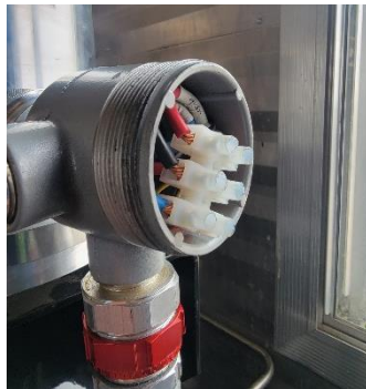
Conductor Cable Termination in Junction Box
