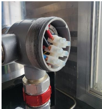
Conductor Cable Termination in Junction Box
